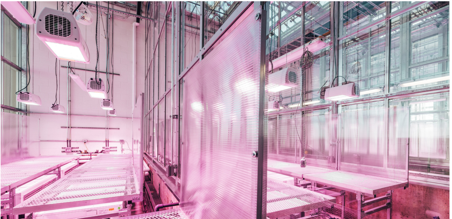
UW Science Initiative - Roof level 12 separate greenhouses totaling 6,400 square feet & two walk-in growth chambers
