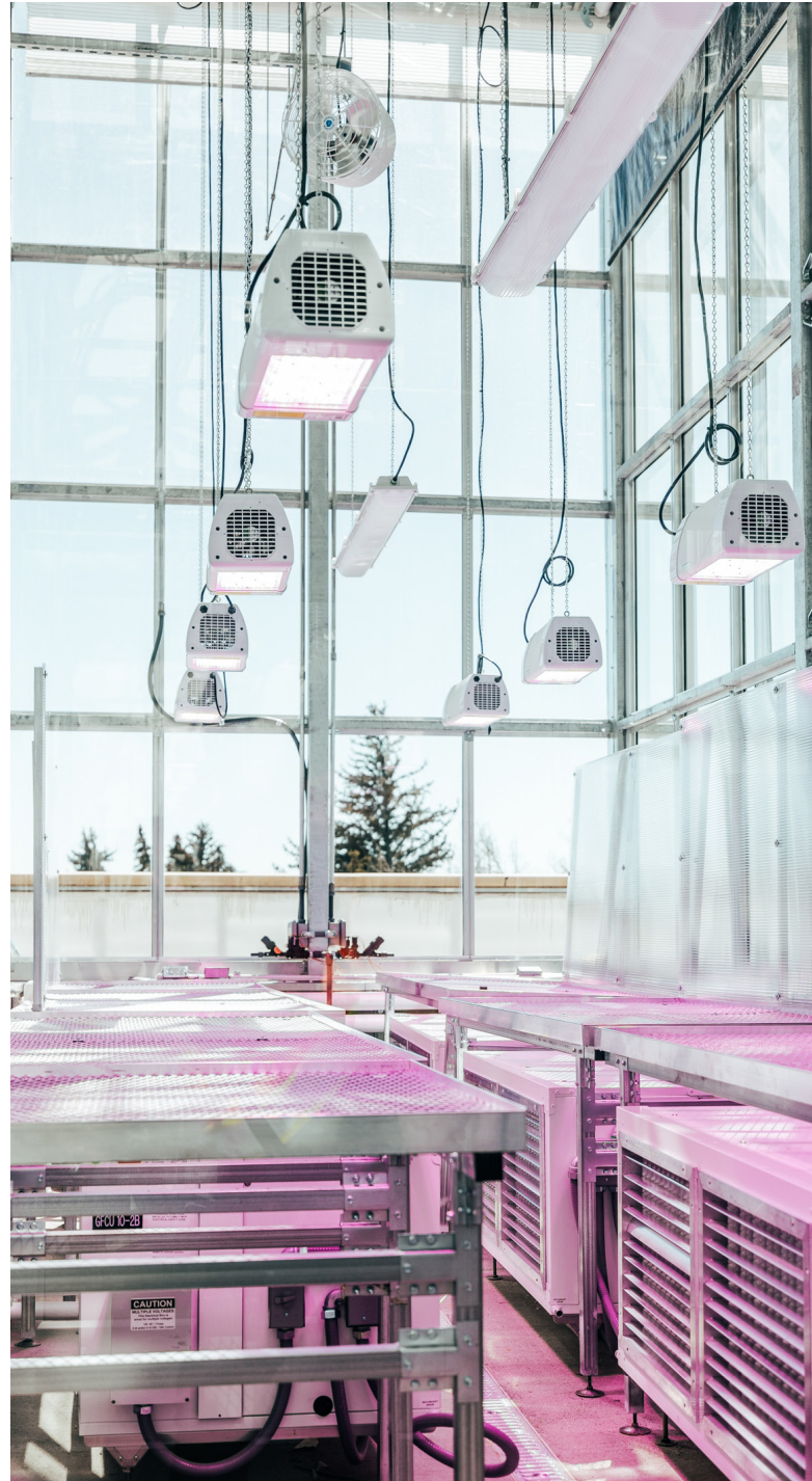
UW Science Initiative - Roof Level Greenhouses
